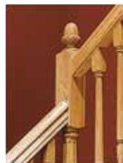
Handrail runs straight into the top block of the newel post at all landings.
